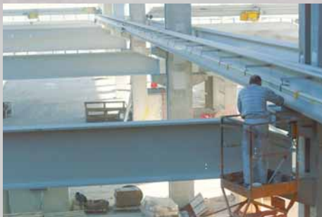
Working at windy heights – lifting platforms were used everywhere to position the cranes' cross beams where they would actually be used later.
